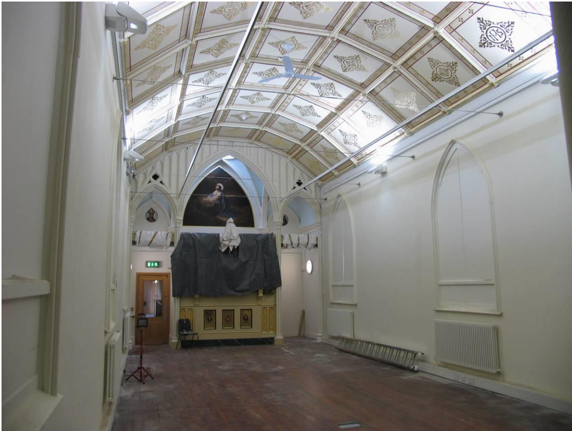
View of the former convent chapel with the reinstated gilded ceiling, restored reardos and oil paintings.
